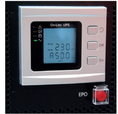
Right: via the central control panel with background-lit LCD display and LEDs the operating status, and warning messages of UPS and module are displayed. Furthermore, directly below the display and easily accessible there is the EPO switch for the emergency shutdown of the consumer.
