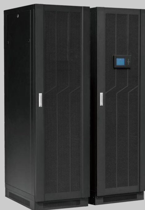
Below: additional cabinet with batteries
